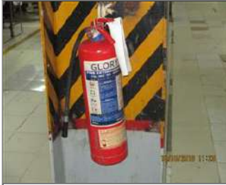
Photo of fire safety equipment Fire extinguisher.JPG
