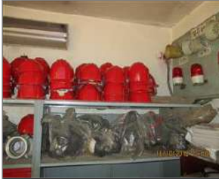
Photo of fire safety equipment Fire equipment.JPG
