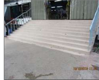
Photo of non-conformity Hand rail at stair_corrected.jpg
