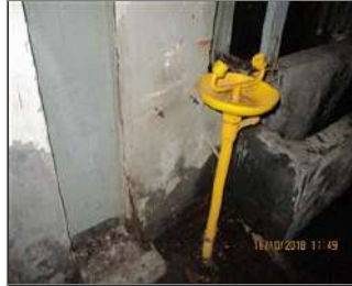
Photo of the inside of the main production hall Eye wash point.JPG
