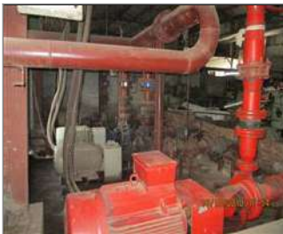
Photo of fire safety equipment Fire hydrant pump.JPG
