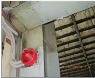
Photo of fire safety equipment Fire alarm.JPG
