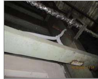
Photo of non-conformity Electrical wiring concealed_corrected.jpg
