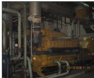
Photo of the inside of the main production hall Generator room.JPG
