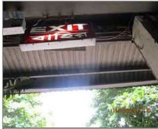
Photo of fire safety equipment Exit sign.JPG
