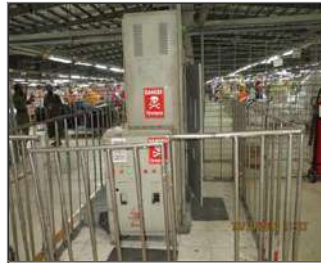
Photo of the inside of the main production hall Electrical distribution board.JPG
